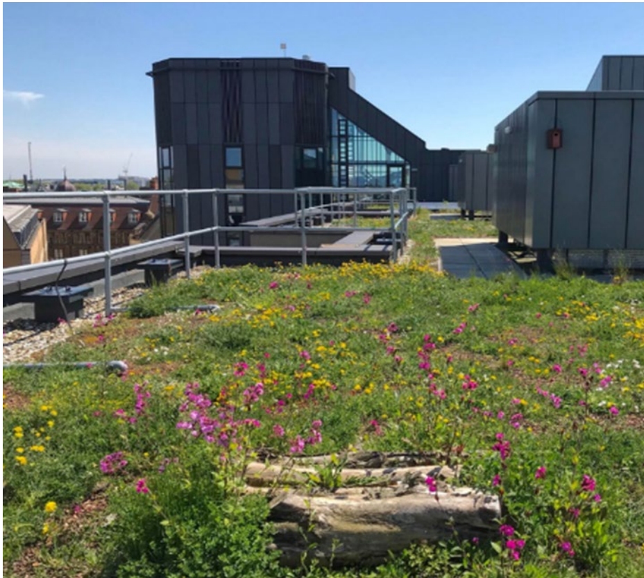
Plate 2: Biodiverse extensive green roof on the David Attenborough Building, Cambridge. Credit: Green Infrastructure Consultancy
